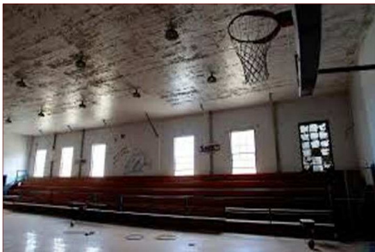
The Belleview Sports Centre gym needs painting.
